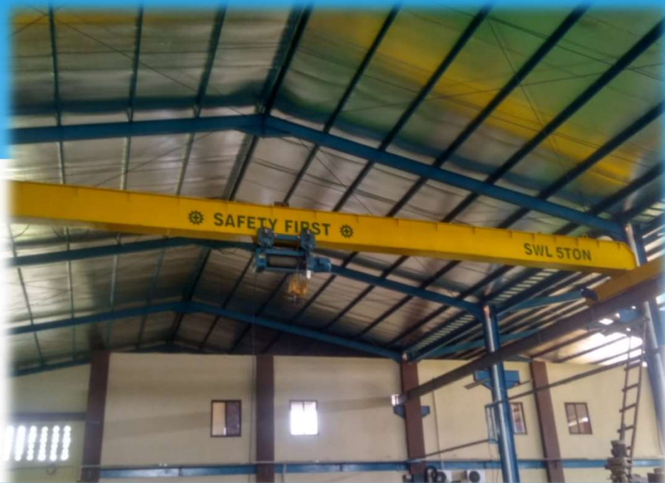
Lifting & Handling Overhead crane SWL 6.5 Ton
