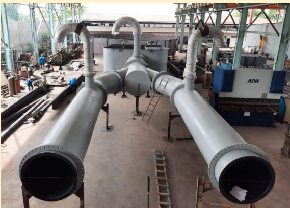
Pipe System (Rubber Lining)
