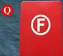
Firehose and cabinet
