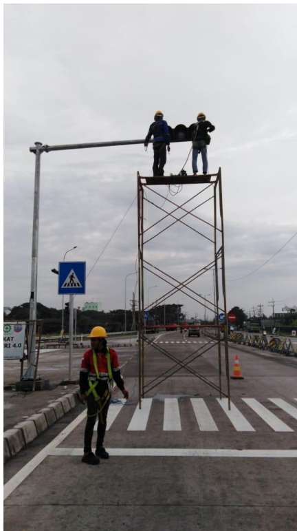
INSTALATION TRAFFIC LIGHT
