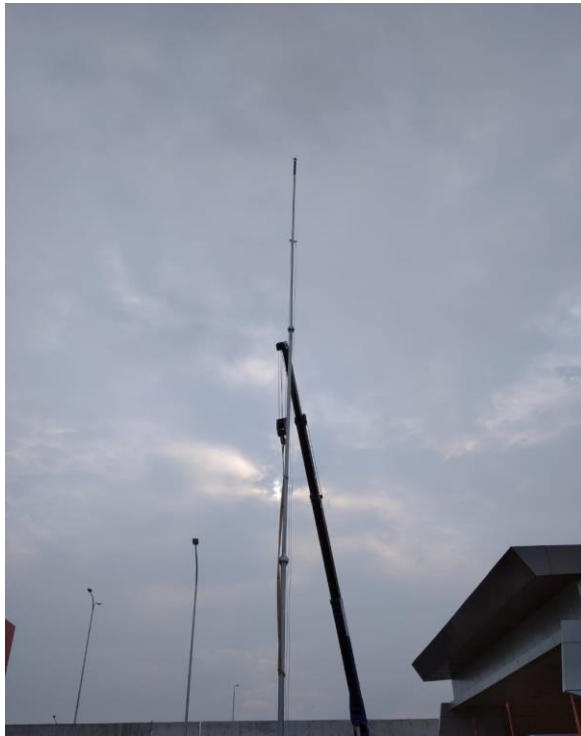
INSTALATION PENANGKAL PETIR
