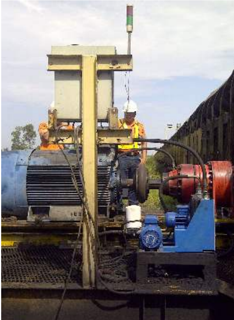
DRIVE JETTY COAL CONVEYOR
