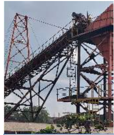
DRIVE COAL CONVEYOR
