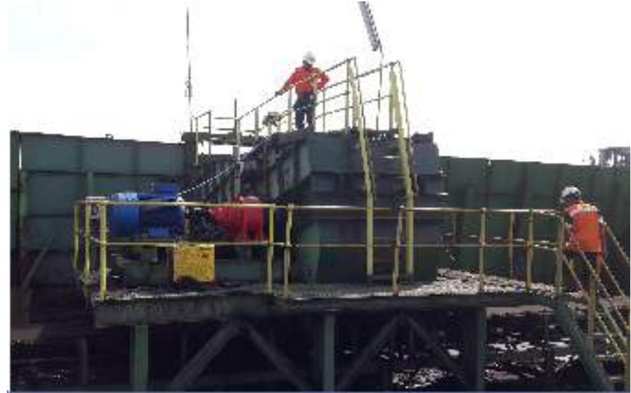
CHAIN FEEDER, COAL CONVEYOR
