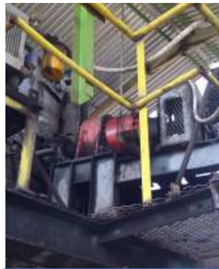
DRIVE JETTY COAL CONVEYOR
