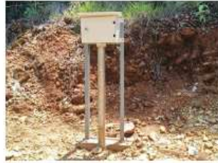
Instalasi Negative Junction Box
