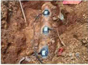
Bonding kabel negative
