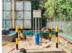
Instalasi Positive Junction Box
