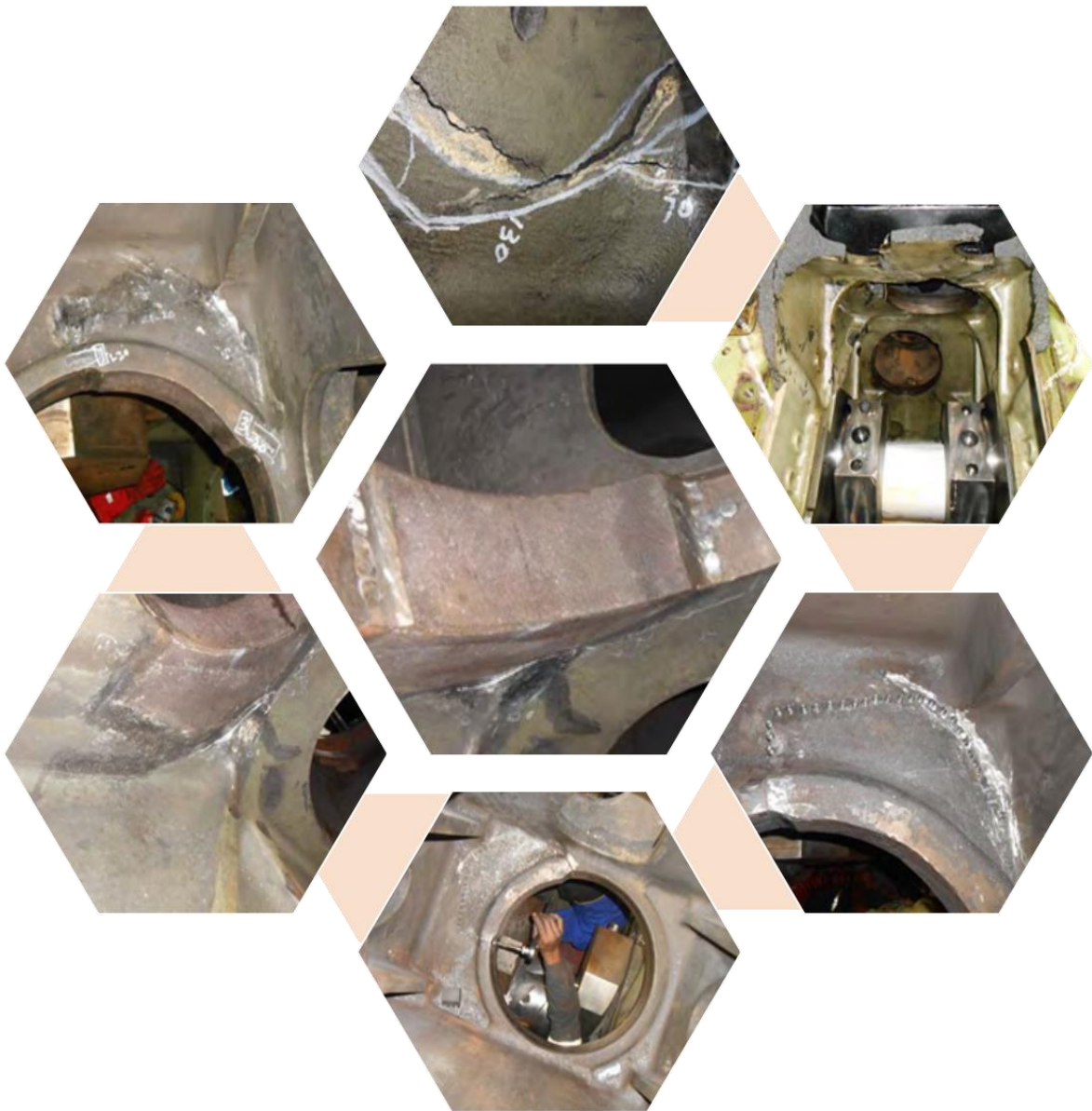
CRACK REPAIR ON ENGINE SULZER ZV12- 40/48 PLTD UNIT KLEDANG
