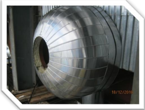
INSULATION BOILER TANK
