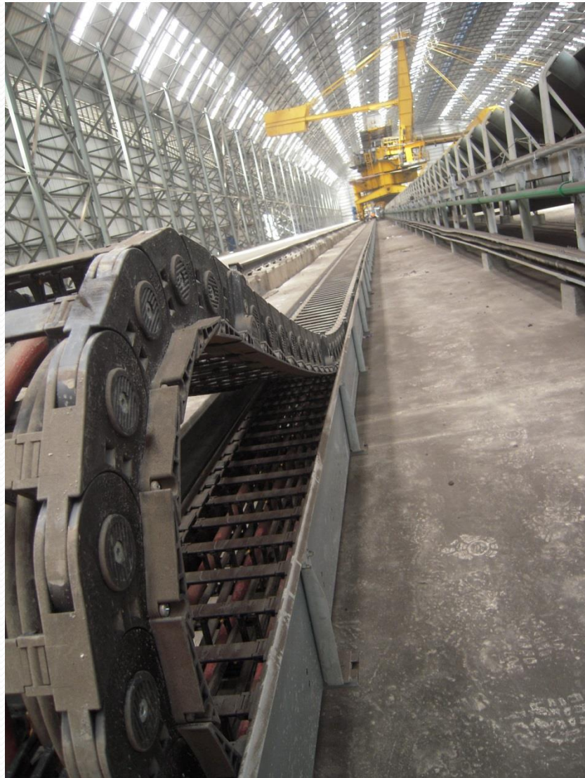
Long travel energy supply system for stacker reclaimer and ship unloader
