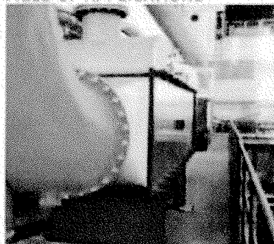
Low pressure vacuum condenser
