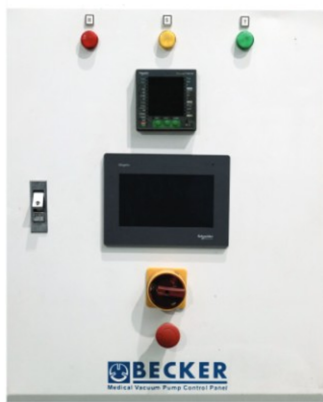
Intidaya Online Monitoring System
