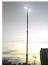
PT. TANTO LINE Depo 4 Jl. Teluk Kumai Pasang Flood Light
