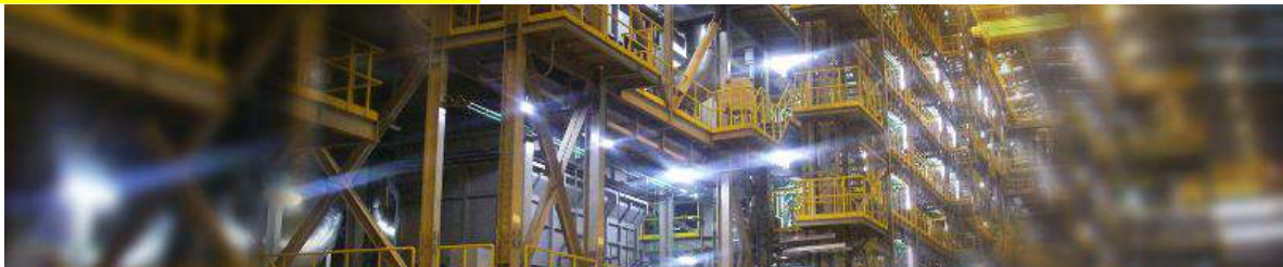
CAL & CGL for Steel Mill
